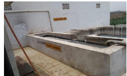
Figure 6: Equalization Tank and Screen Chamber
